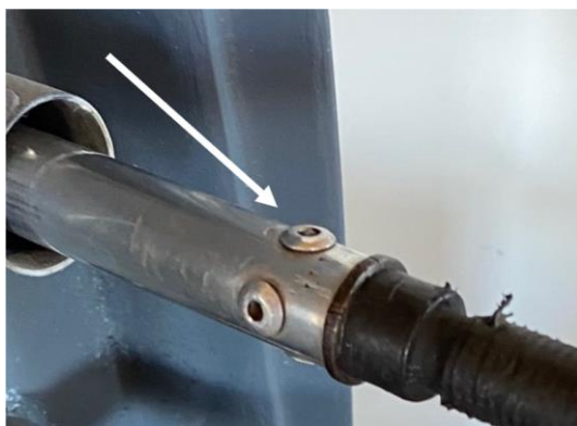
Picture 1: Installation situation old fittings
